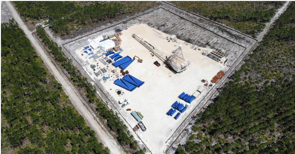
TPM broke ground on staging areas before obtaining required permits. (© Joseph Kelly, Georgia River Network)
